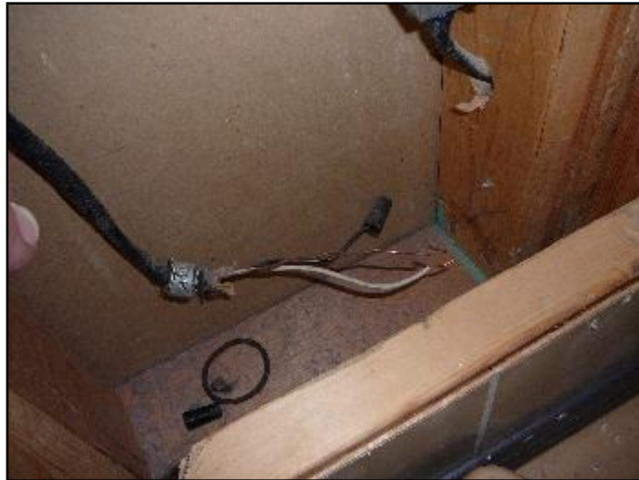
provide proper termination
