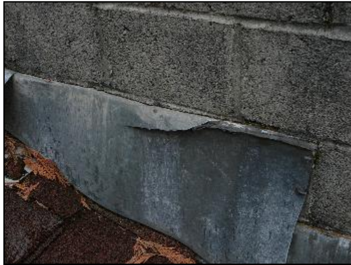
damaged- replace when roof replaced
